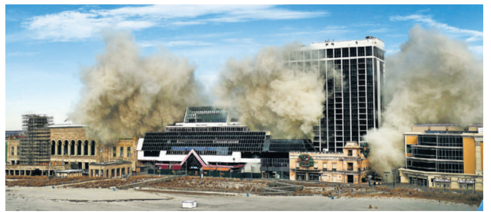
The 39-story main tower of the former Trump Plaza hotel-casino in Atlantic City is imploded Wednesday. The site shut down in 2014. Michael Mancuso, for The Star-Ledger
